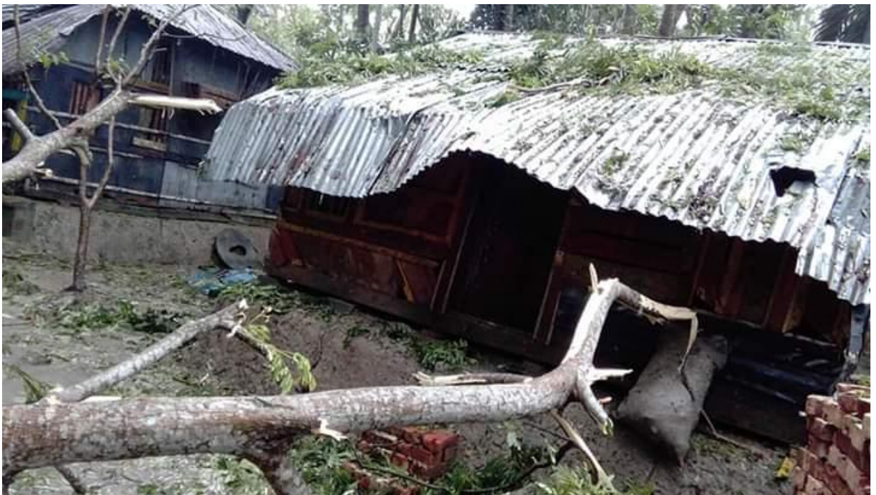
Figure: A damaged house in Mongla (Photo taken by MahmudulHasan, JJS)
